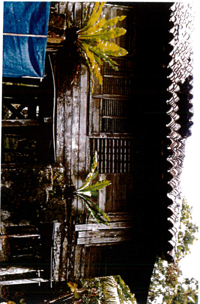
Another view in the right side of the structure. As shown is the extension part of the structure that rests in sturdy wooden columns.
