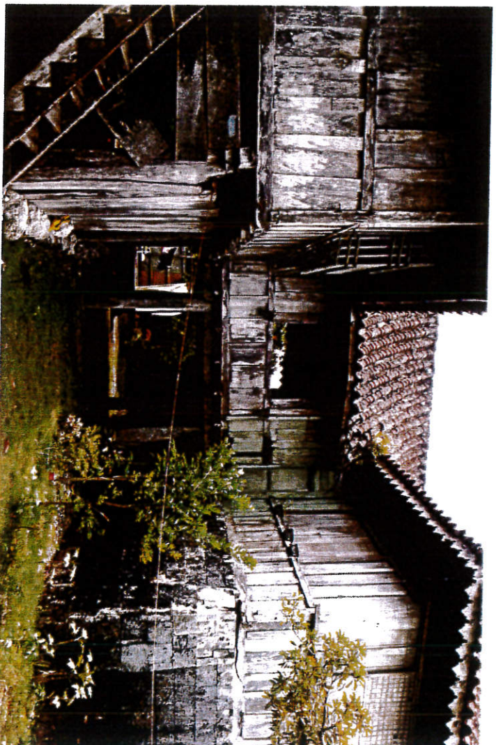
Another view in the left side portion of the structure. Strong depiction of bahay na bato structure. Evident use of wood in the structure.
